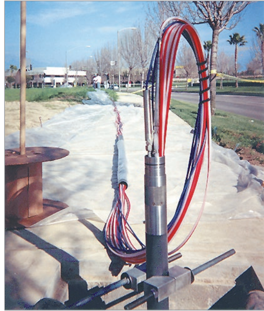
Contaminant investigation at a U.S. Air Force Base. Waterloo Systems installed to 700 ft. in overburden using screened and cased wells. Up to 6 zones per hole with dedicated pumps and transducers.
