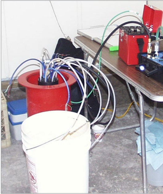
Four Waterloo Systems were installed to monitor a chlorinated compound release. Systems were installed at depths ranging from 430 ft - 750 ft, with most monitoring 7 zones. The Ports were constructed with both Double Valve Pumps and Vibrating Wire Transducers.
